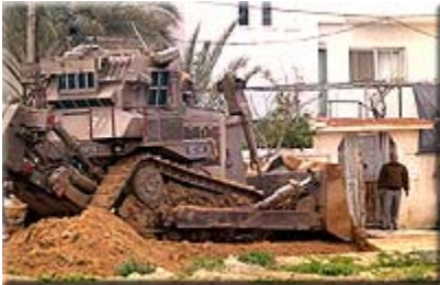
A man's home about to be destroyed by an American supplied bulldozer. In many cases the drivers will not even allow the family to take what they can carry, or leave the building before they begin demolishing it. Usually there is no warning.
