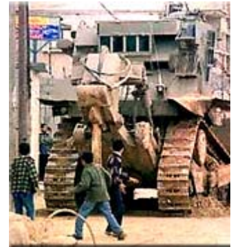
October 2002: Bulldozer erasing another house in a RAFAH neighborhood PHOTO: MOHAMMED OF RAFAH
